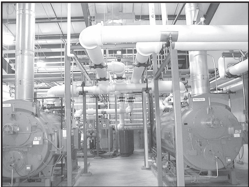
Boiler System within CT Valley Juvenile Center Cogeneration Plant
