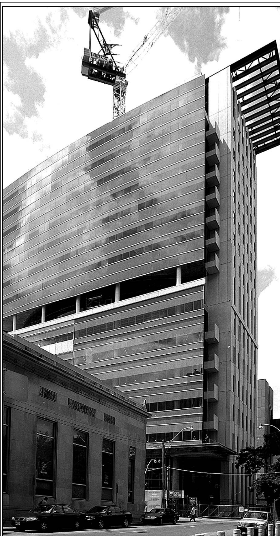
QUEEN STREET TOWER - Work continues at 180 Queen Street West for the Canada Life Tower office building in Toronto. Construction manager EllisDon Corp. began the 15-storey office in December 2003 and completion is scheduled for this December. There will also be four levels of underground parking. The project was designed by Kuwabara Payne McKenna Blumberg Architects. Consultants are: Yolles Partnership Inc. (structural); The Mitchell Partnership Inc. (mechanical); and Mulvey & Banani International Inc. (electrical). Subcontractors include: Active Excavating; Deep Foundations Contractors Inc. (shoring/caissons); Res 2000 Structures Inc. (formwork/concrete supply); Res Precast Inc. (precast); Harris Rebar (rebar supply); Limen Masonry; Urban Mechanical Contracting; RE Wilson Electrical Contractors (2000) Inc.; Sota Glazing Inc. (windows); Bothwell-Accurate Co. Ltd. (roofing); Tedesco Waterproofing Inc.; and ThyssenKrupp Elevator Ltd.
