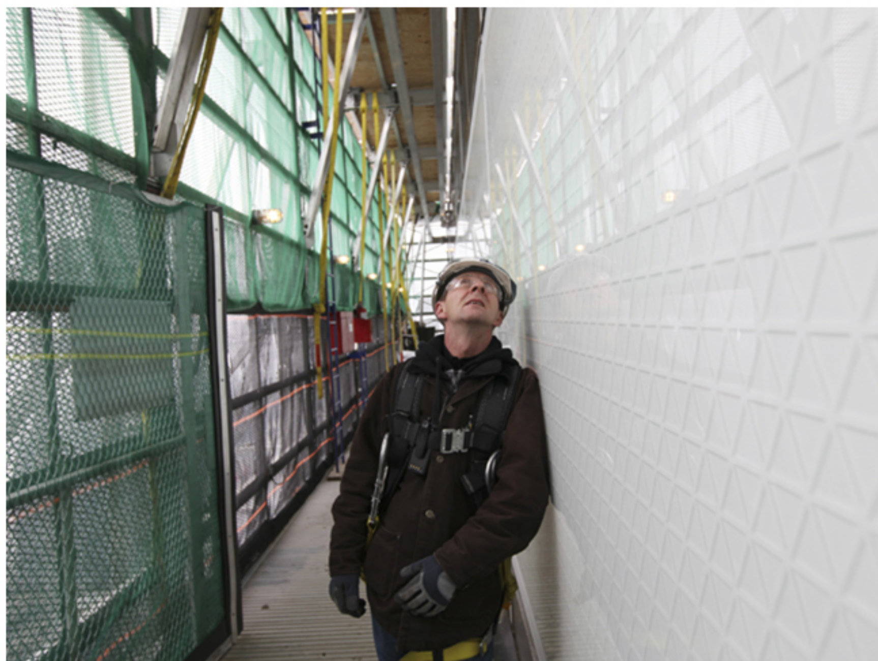
Michael Brodigan examines a panel on the suspended elevated platform, which construction crews are using to replace the marble cladding with glass panels at First Canadian Place. Tyler Anderson/National Post
