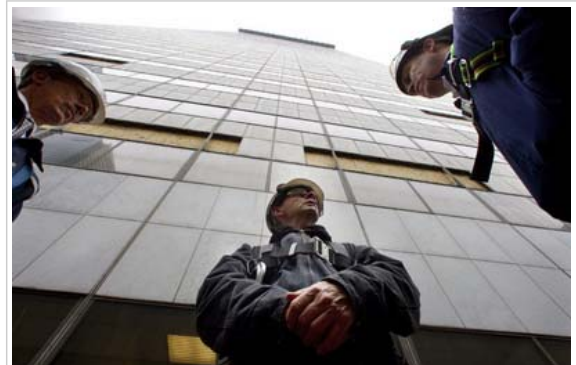
Jim White, V.P. construction, Brookfield; Mike Brodigan, construction manager, Ellis Don and Pat Crosbie, of Atlantic Hoisting, are framed by First Canadian Place, which is undergoing a dramatic makeover as all the marble tiles are removed and replaced with triple layer glass sheets. May 18, 2011.
